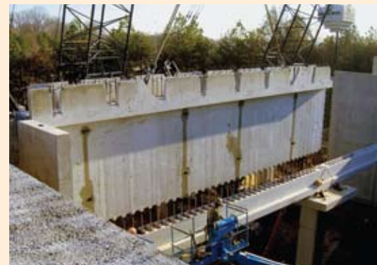
The beams for the Howell Mill project were created in pieces that were then assembled on site.
